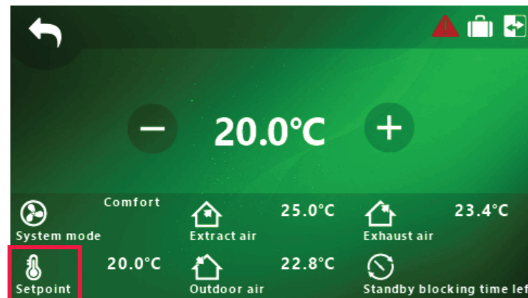
Fig. 5.6.1.4 ST-SA-Control and SALDA AIR temperature setpoint screen view
